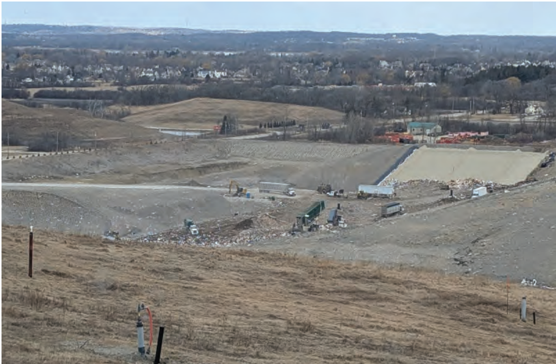
New lift in Phase 3
